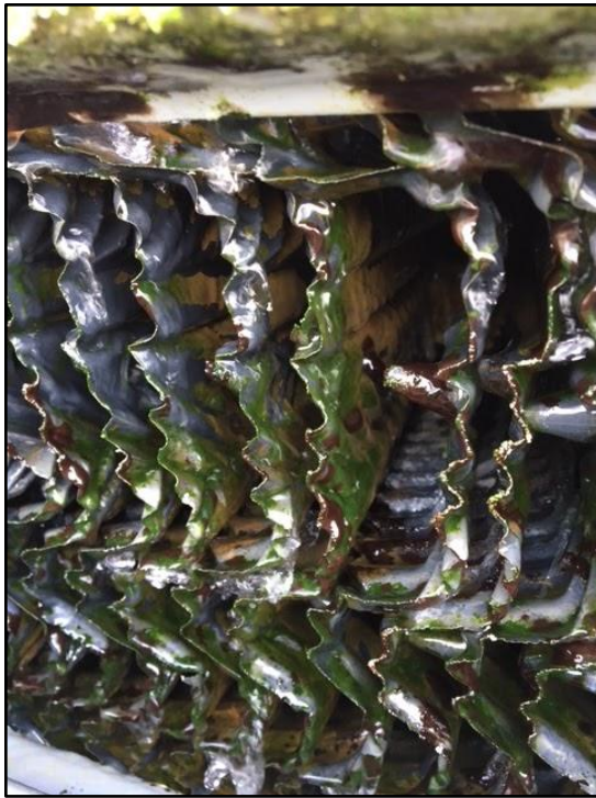
Before: Fill showing algal/ biofilm deposits/growth
