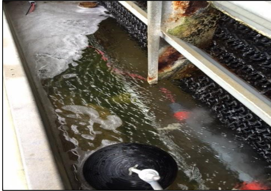
OzoPen placed in Cooling Tower sump. Note bubble diffusion in water
