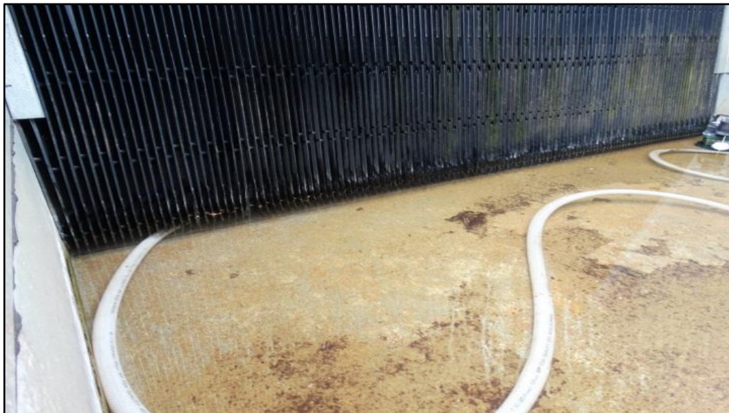
After: Note flex hose of filter pump used to remove oxidized particulates
