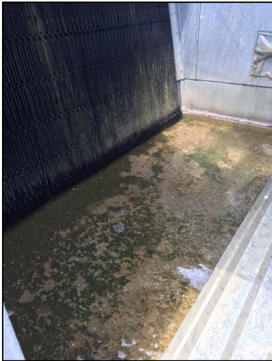
Before: Algal deposits on floor of sump- air side
